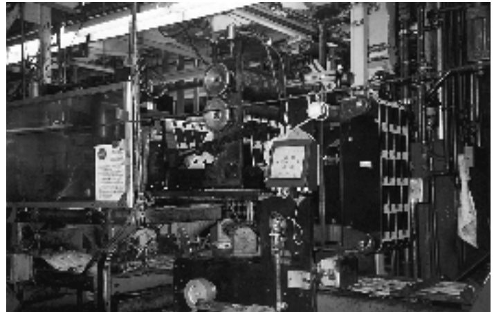
91 synchronous drives and 2000 I/O points control Polaroid's flat battery manufacturing line.
