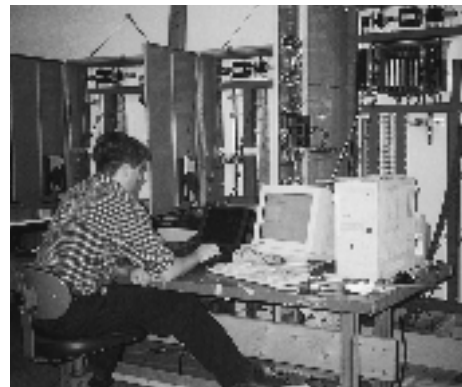
Bob Patrick of Superior Controls tests the gas turbine control system consisting of four PLC enclosures.
